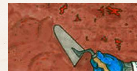
5. Brush the plaster with a trowel to close all gaps even small ones . Then scratch the plaster to facilitate the adhesion of next layer.
