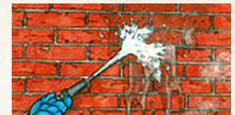
3. Wash or pressure wash the affected surfaces to remove loose bits, grease and salt residues from the surface.
